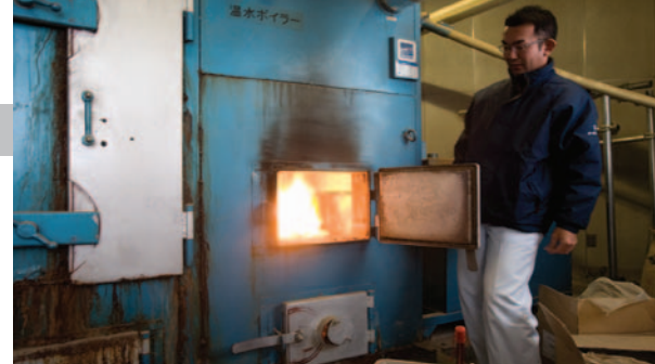
This pellet boiler heats...
