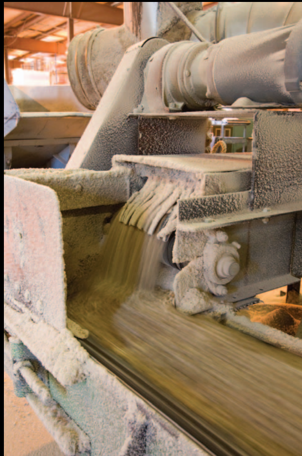
Pellet mill open for business at 4 tons per hour
